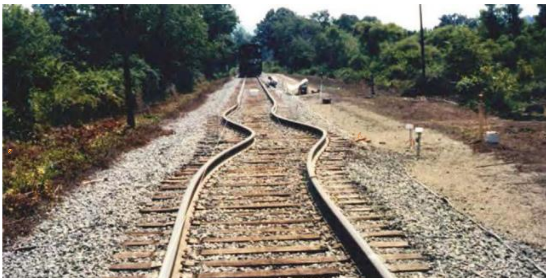
Fig.1: Track Buckling (US Department of Transportation 2015)
